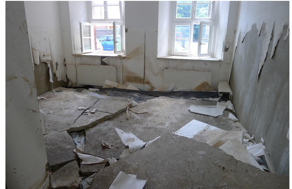
Schäden an Zementestrich (Goltz 2013)
