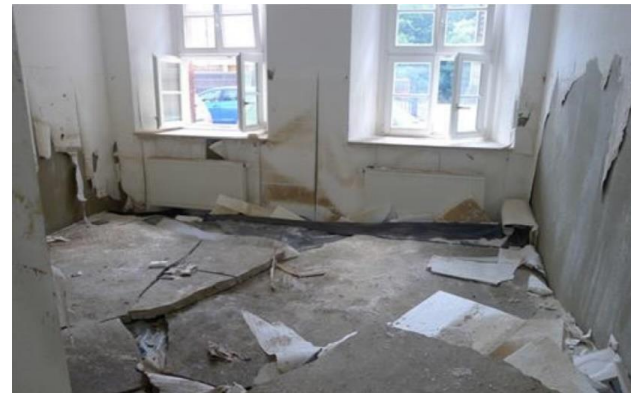
Schäden an Zementestrich (Goltz 2013)
